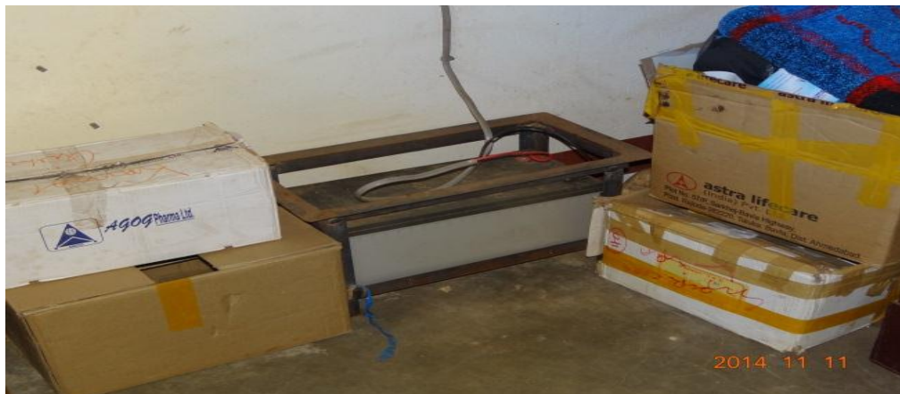
Battery not in protective cover at Dr Oryang SS in Oyam district
